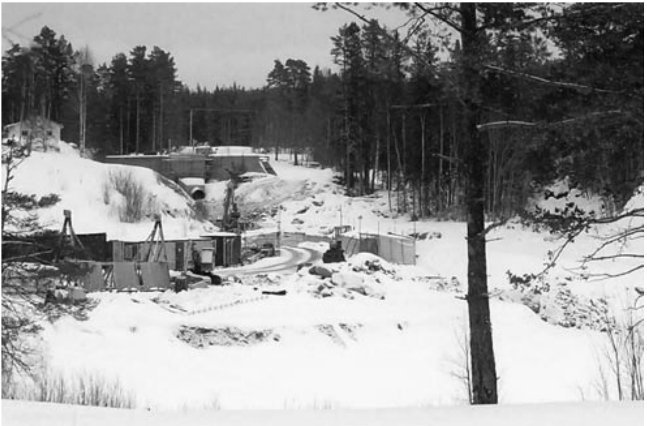
Ljung River mini power station under construction on the Ljung River, Bräcke municipality in central Sweden. Capacity 1,200 kW, dimensioned water discharge 9 m 3 /s. The concrete dam that will force the water to flow through the turbine of the power station can be seen in the background. The river is hidden behind the cover in the centre of the picture. At the very right the river is visible but covered with ice. Photo: Hans Isgren
